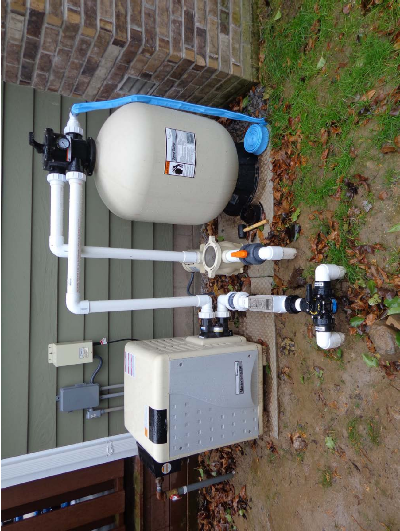
Example of Pool Filter & Heat Pump
